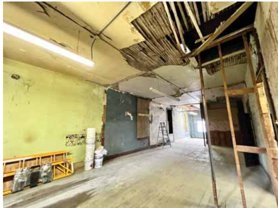
This is part of the second floor of the building local architect and business woman Rachel Mondt wants to turn into apartments.
